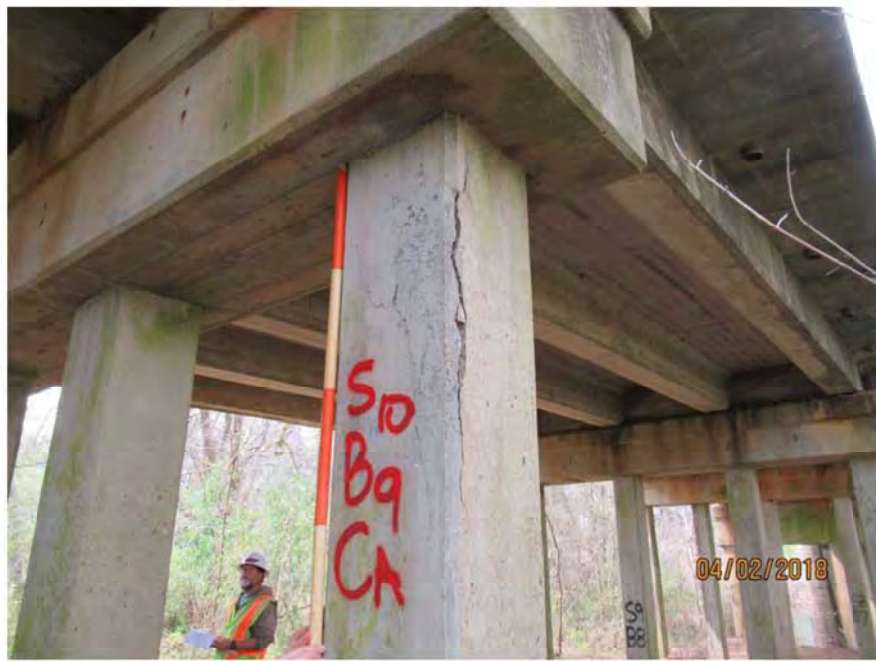
SPAN 10 - BENT 9 - COLUMN A - SPALL/DELM
