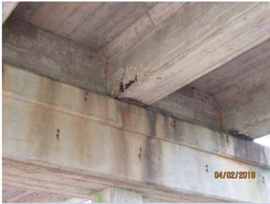
SPAN 9 - BENT 8 - BEAM B - REBAR SPALL
