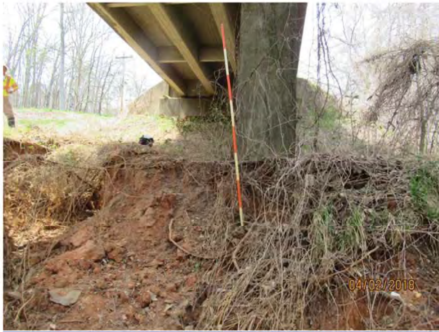
SPAN 2 - BENT 1 - COLUMN A - EROSION
