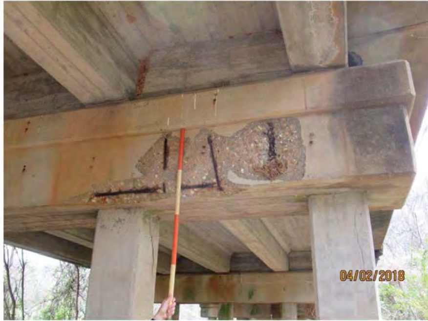
SPAN 9 - BENT 9 - BETWEEN COLUMNS D & E - REBAR SPALL
