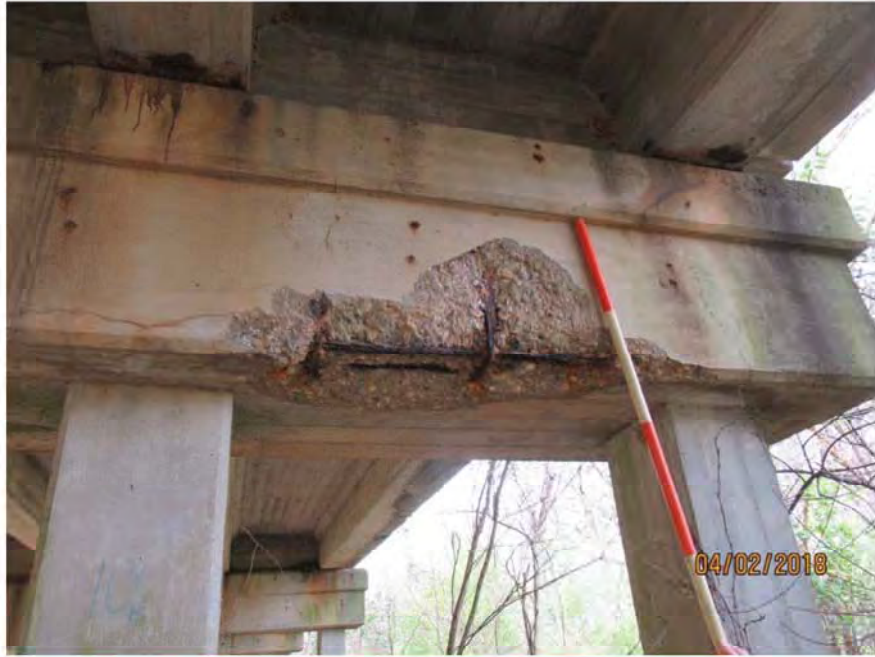
SPAN 11 - BENT 10 - BETWEEN COLUMNS A & B - REBAR SPALL
