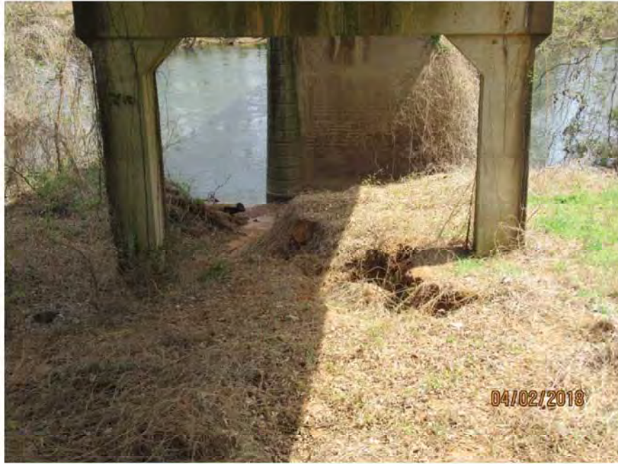
SPAN 1 AND 2 @ BENT 1 - EROSION
