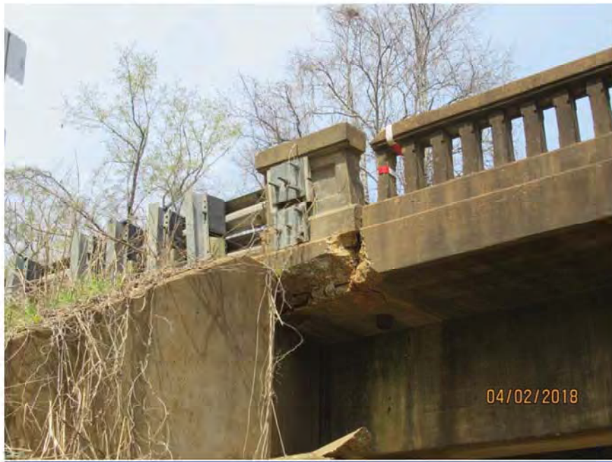
APPROACH 1 - RIGHT - RAIL DAMAGE
