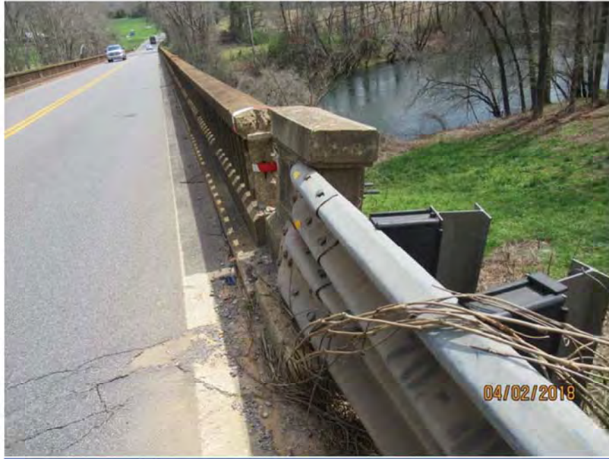
APPROACH 1 - RIGHT - RAIL DAMAGE
