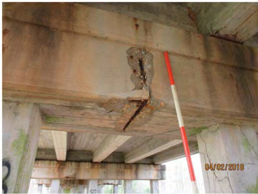
SPAN 13 - BENT 12 - BETWEEN C AND D - SPALL
