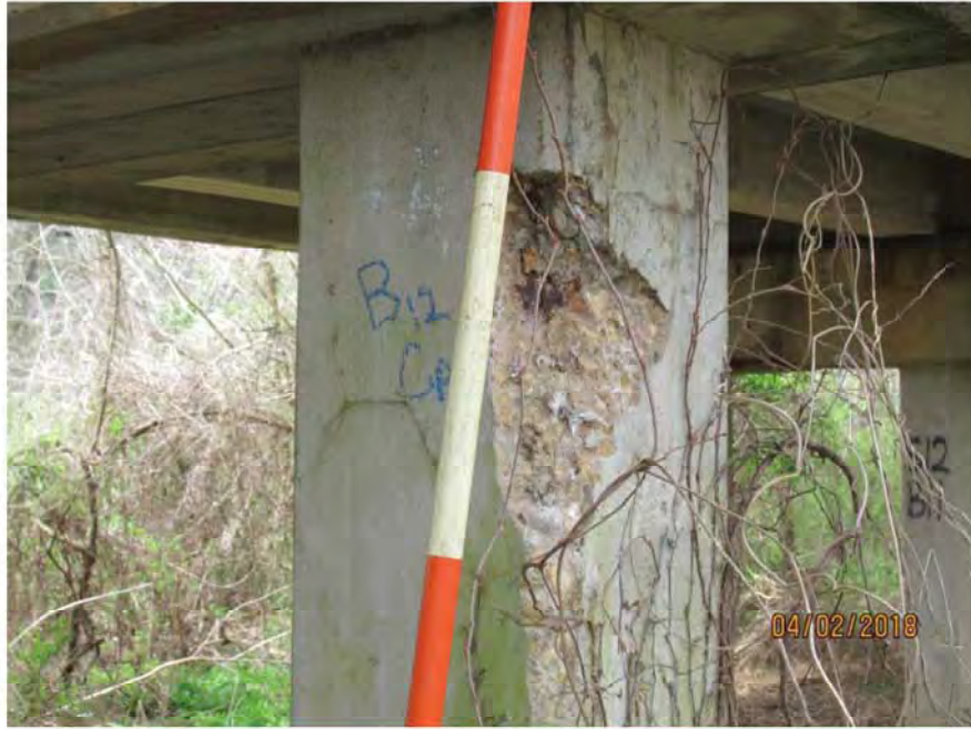
SPAN 13 - BENT 12 - COLUMN A - SPALL
