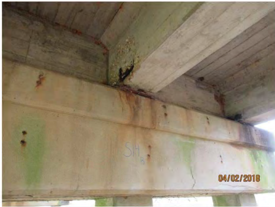
SPAN 14 - BENT 13 - BEAM B - SPALL
