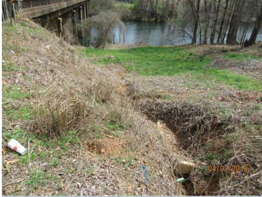
APPROACH 1 - RIGHT - EROSION
