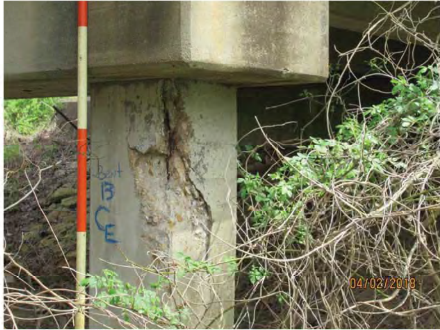
SPAN 13 - BENT 13 - COLUMN E - REBAR SPALL
